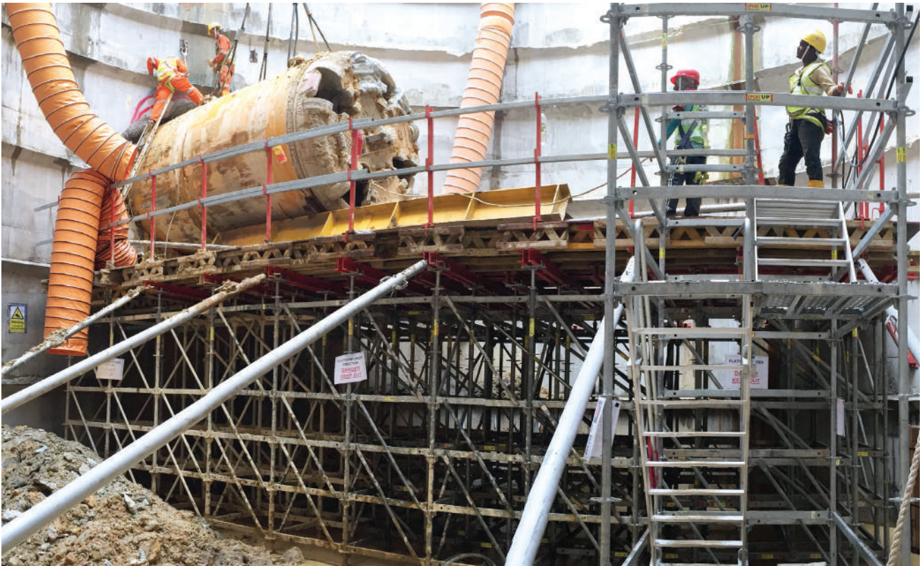
PERI products resist high pressure on the construction site. The dismantling of the TBM was carried out on top of the temporary platform of PERI.
