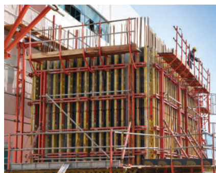
A liftcore for both cargo and passengers lift were seen using the PERI CB 240 Climbing Formwork system.
