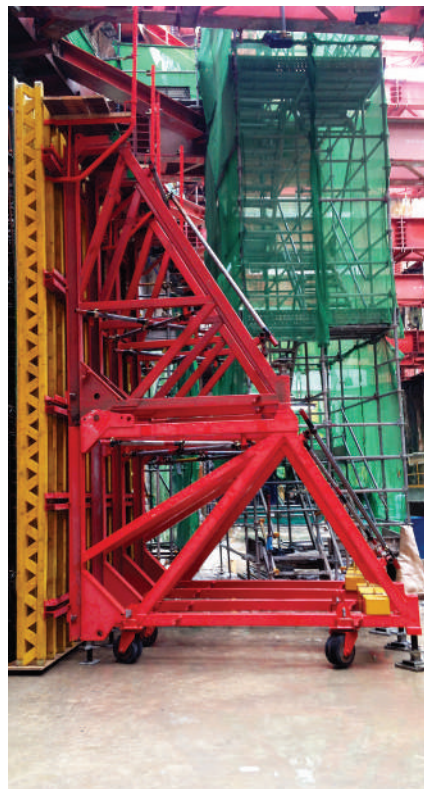
SB Brace Frames and VARIO GT 24 Wall Formwork for casting of walls.
