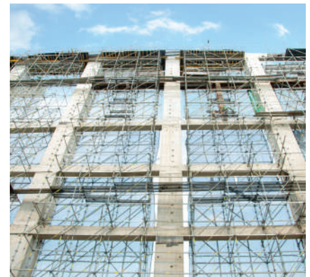
PERI UP Rosett shoring system managed to carry loads of 1.2 m-deep beams at height of 35.55 m.
