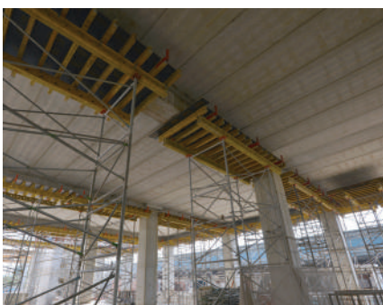
An overview of the PD8 Table system being used to support the beam of the warehouse.
